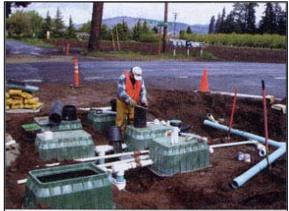
Final construction work on a distribution manifold for a fully pressurized irrigation system funded with surplus hydropower revenue. The pressure pipe system replaces archaic, inefficient irrigation canals.
