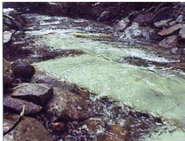
The Gate Creek horizontal screen, an innovative horizontal screen system in place at the Gate Creek diversion, a small source of water for both hydropower and reservoir storage for irrigation and recreation.
