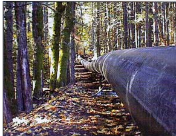
Large diameter HDPE installation: replacing an inefficient (and ecologically unsound) hydropower and irrigation supply canal with large diameter highdensity polyethylene pipe. The pipe project was funded with surplus hydropower revenue.
